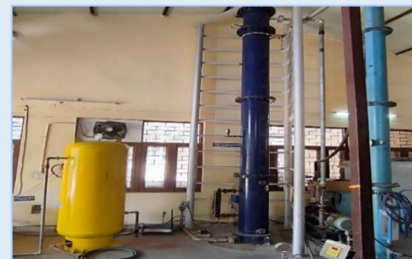
Biogas enrichment and bottling facility at IITD
